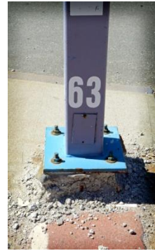
Crumbling concrete due to storm, water erosion and salt damage.
